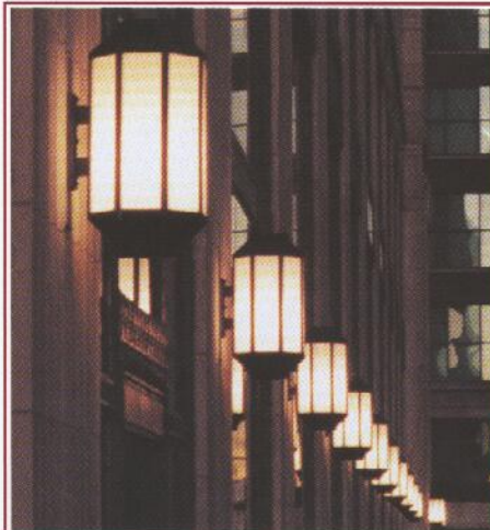
SHOWN IN PHOTO: 29091B LUMINAIRE WALL BRACKETS. Merchandise Mart - Chicago, IL
